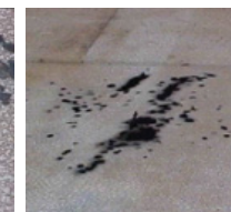
Roof Holes in an AST
