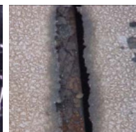
Corrosion on a Support Beam
